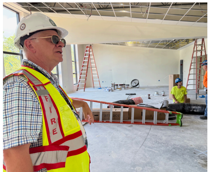
Roger Hooper during construction of the York County Regional Training Center in Alfred. Photo: Tammy L Wells
